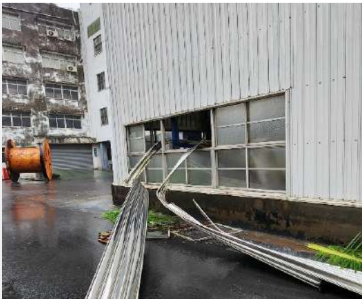
Damaged north-side windows of Power Plant 3
