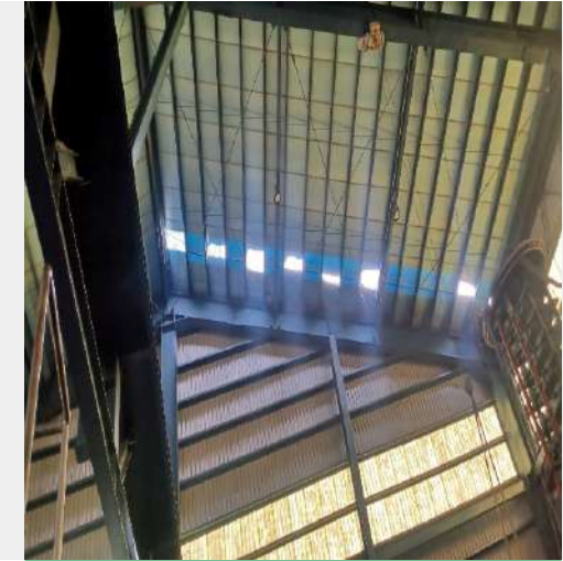
Damaged roof of the inspection building
