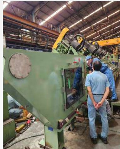
Replacement of oxygen-free copper idle rollers.
