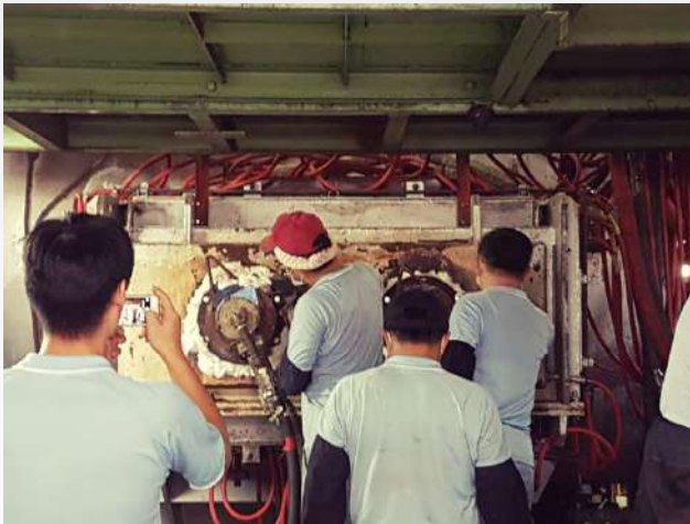
Upgrade of the oxygen-free copper induction furnace.
